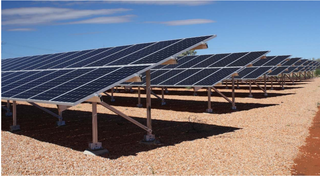
Photo 1. Example of a typical fixed tilt system
